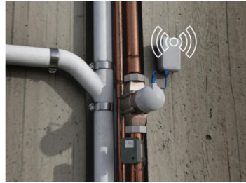
Leak Detection System
